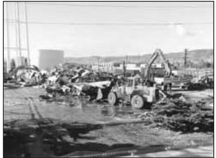
One of the structures demolished in fiscal year 2002 is Building 125 (above). This building formerly was a laboratory used for calibrating equipment, among other things.
