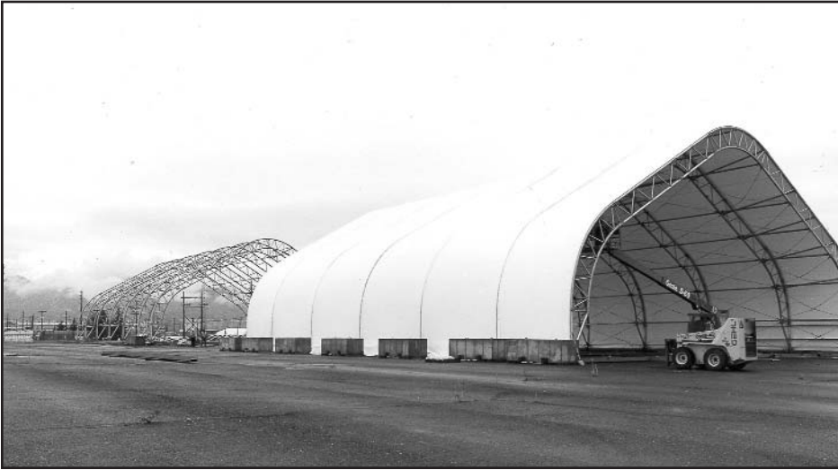
Construction of the protective tent over the 903 Pad is shown above. Work on removal of the asphalt pad began in mid-November.
